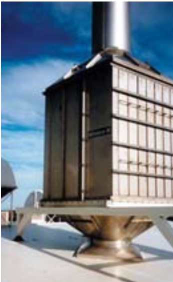
Special stainless steel splitter attenuator with removeable splitters installed at a Southland dairy factory
